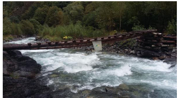
A bridge on Asa River, near the confluence of Taniestskhali and Asa
